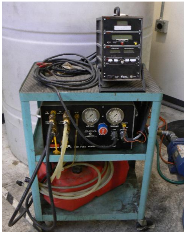
Figure 20: Fuel Conditioning/Metering and Display Units
