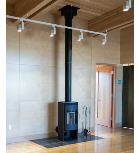
Above Pellet fire place offers a practical solution to heating the flex space that is not only a homage to Idaho forestry products but also a fitting aesthetic focal point as you enter the building.
