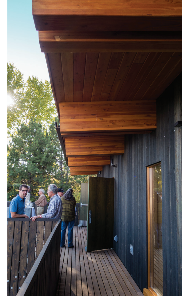
Above Five foot overhang showing off exposed roof structure and T&G soffit. The contrast of the rich natural wood color with the dark wood stain shows off the aesthetic versatility of wood.
