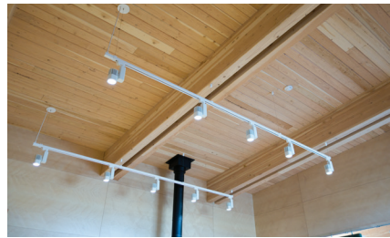
Above Energy efficient LED track lighting doesn't impede the lofty feel and adds an elegant touch of spot lighting.
