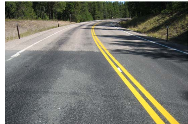
Condition 1 year after application
