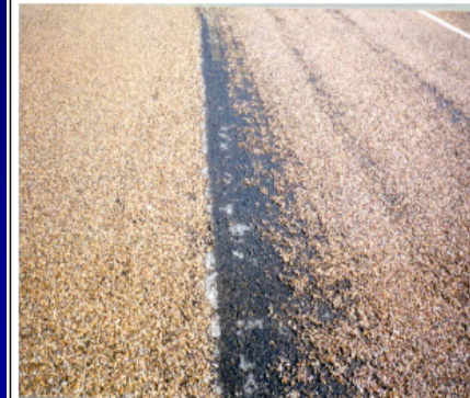
Condition: Cover Material Loss Attributed to Insufficient Embedment.
