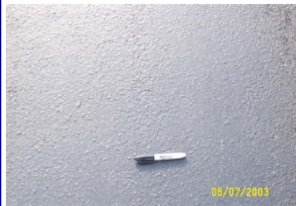
Condition: Heavy Tracking, Bleeding
