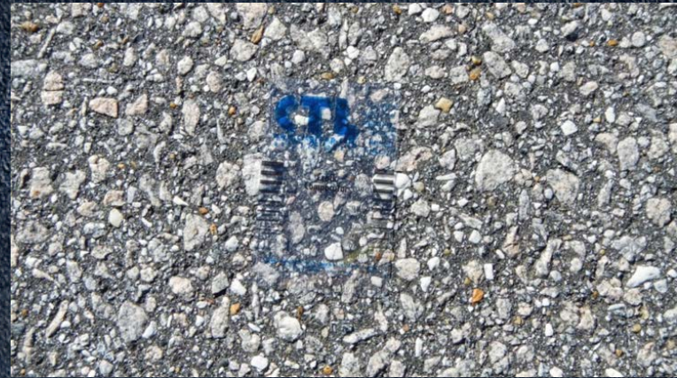
45% RAP PG 52-28 Crack
