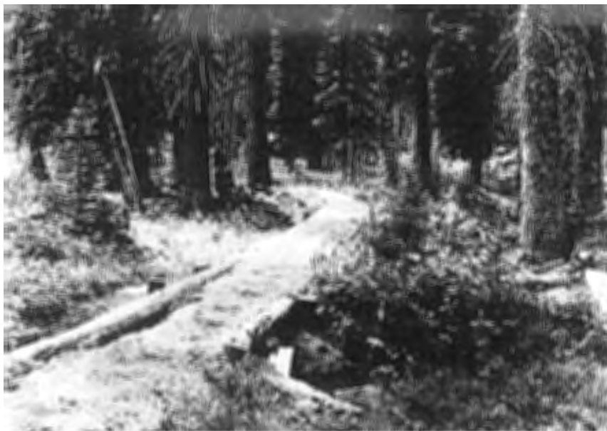
FIGURE 7. Turnpiking can be used to elevate sections of trail above surrounding wet areas. The trail surface is sand held in place by log stringers. Culverts allow water to pass beneath the trail. (Photo: D. N. Cole.)
