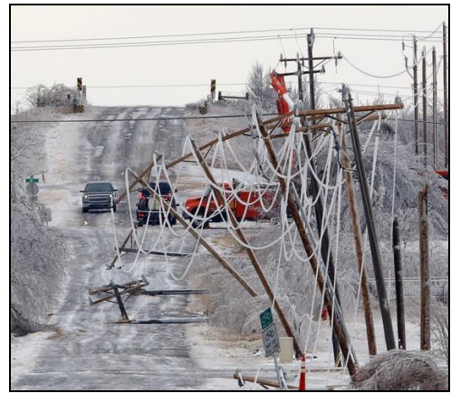
Figure 1. Weather-induced power line damage.
