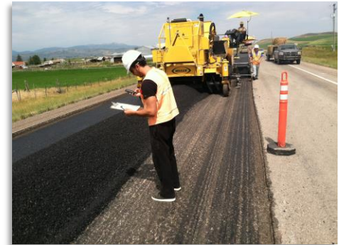
Graduate student Ahmed Muftah checks the mix temperature during construction of the fiber project on US-30
