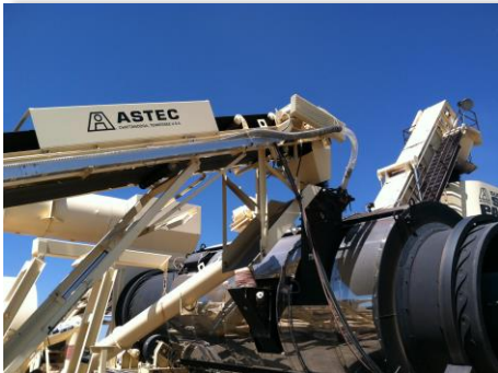
Process of injecting fibers into the mix via the Recycled Asphalt Pavement (RAP) inlet of the drum dryer in the asphalt plant
