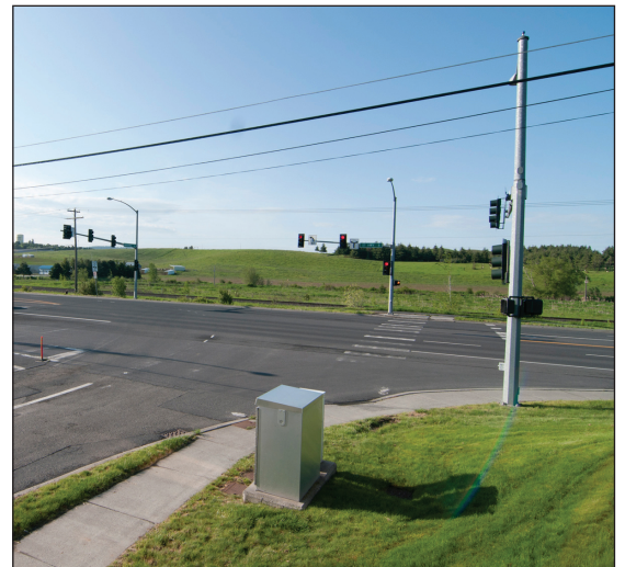
Figure 15. Cabinet housing traffic controller
