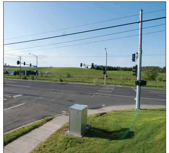
Figure 15. Cabinet housing traffic controller
