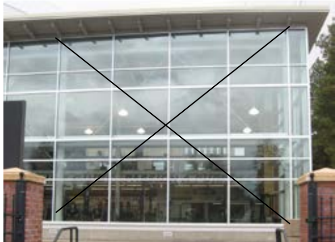
One of the curtain wall bays denoted by the black X with 5 vertical and 5 horizontal mullions. You can see the structural columns behind the first and fifth vertical mullions.
