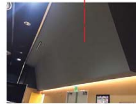
03 Angular dry wall Angular dry wall distributue at the back side of the rppm
