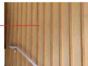
02 Wood absorb panels Distribute along the stage, with soft material in between
