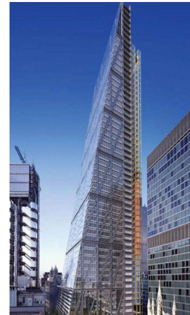
1.7 The Leadenhall Building by Pritzker-prize winning architect Richard Rogers is under construction. It is slated for completion in 2012.
