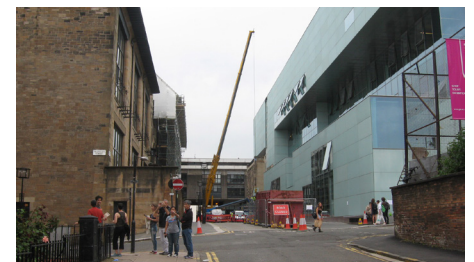
2015—From the corner of Renfrew and Dalhousie—Mackintosh Building standing on left, Reid Building under construction on right.
