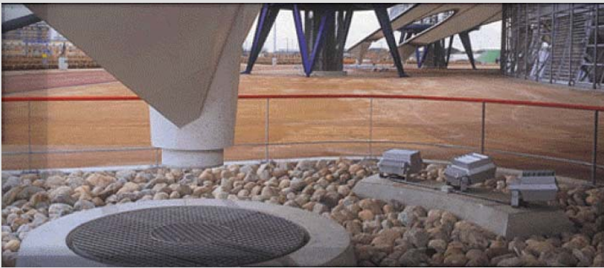
CHP Plant on the Site
