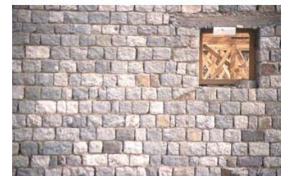
4.05 Mud brick inner walls (t) with granite block facing (b) are stable and made of local materials.
