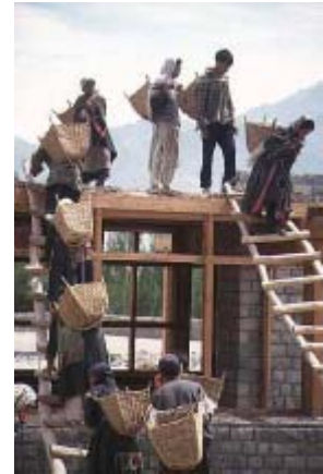
5.4 Arup designed the project to work with local construction crews. CAROLINE SOHIE, ARUP PLUS ARUP ASSOCIATES
