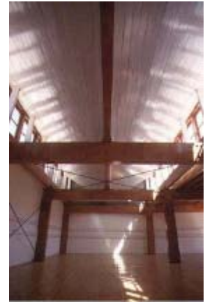
5.8 The splayed roof acts as an indirect daylight source in the classroom. Note the lack of electric luminaires. CAROLINE SOHIE, ARUP PLUS ARUP ASSOCIATES
