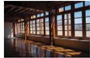
5.6 School rooms feature southeast-facing direct gain windows that ensure early morning warm-up in Shey's sunny climate. CAROLINE SOHIE, ARUP PLUS ARUP ASSOCIATES
