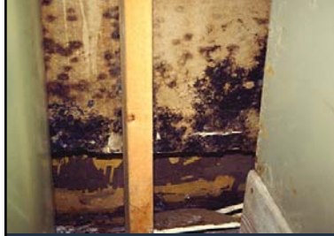
Mold growth on water-damaged interior wall
